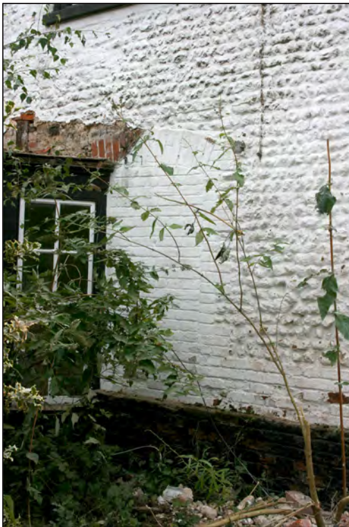
Plate 7. Blocked window beside bay window
