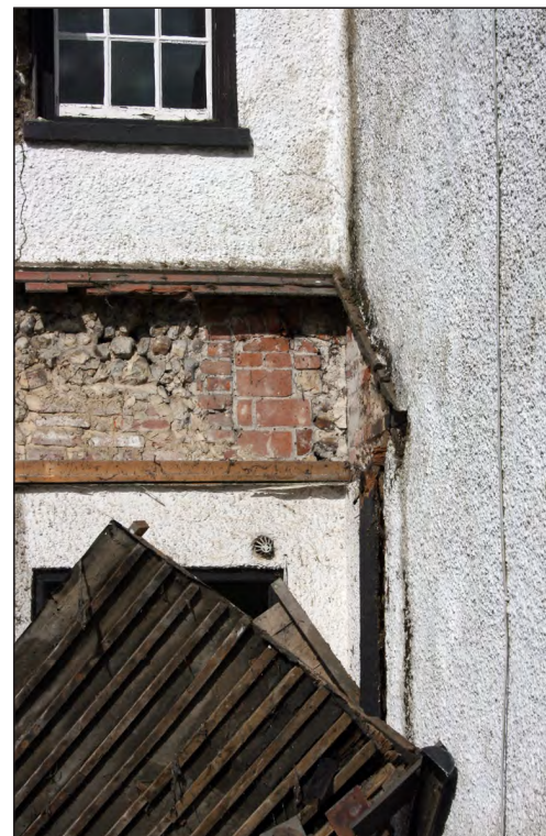
Plate 30. Blocked opening on southern elevation of Building A
